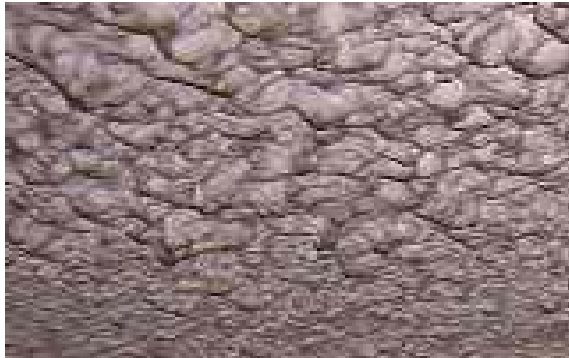
Figure 8: Asbestos sprayed 'Limpet' coating
