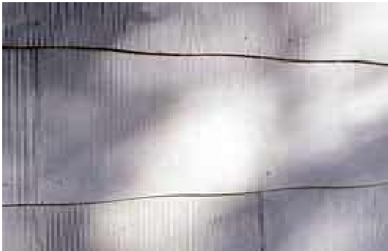
Figure 7: Sheeting (galbestos) containing asbestos
