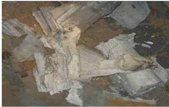
Figure 6: Asbestos thermal insulation debris (contamination)
