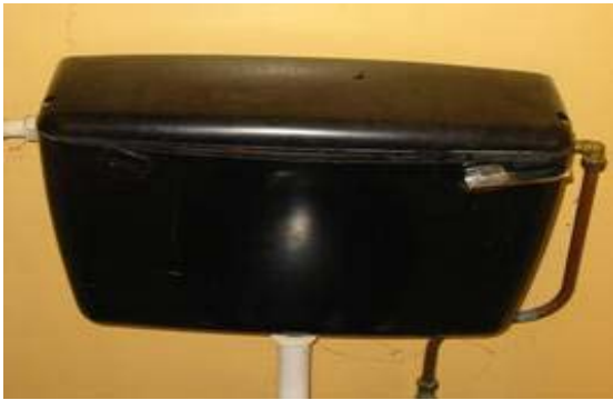
Figure 5: Bakelite toilet cistern containing Bonded asbestos
