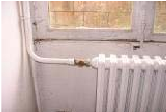
Figure 10: Asbestos panel behind radiator
