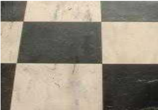
Figure 9: Asbestos thermoplastic floor tiles (Asbestos is often found in the Bitumen adhesive beneath tiles)
