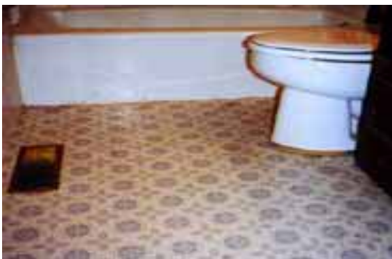
Figure 3: Floor Vinyl (with Asbestos Paper Backing)
